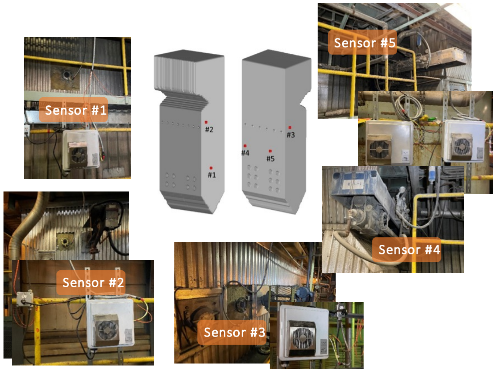
Figure 6. Five mMPMS installations at Basin Electric’s Leland Olds Station Unit 1.
